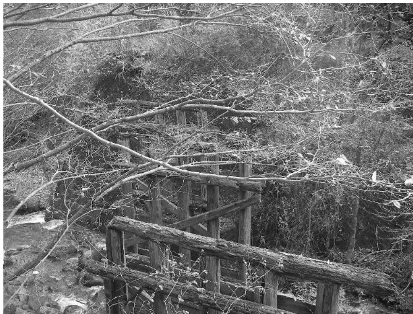
Figure 4 Remains of the bridge over the river upstream from the waterfall of autumn leaves
